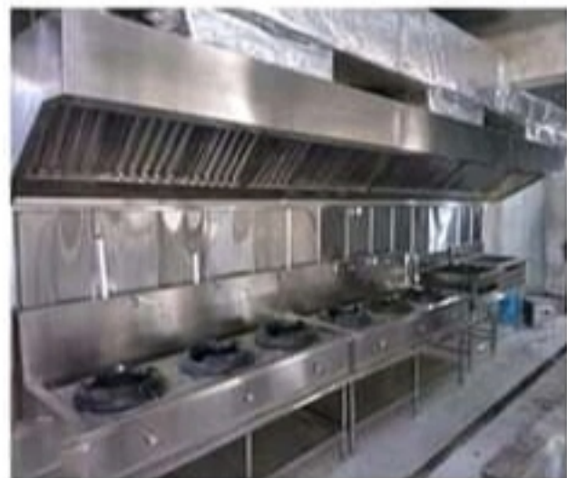
Kitchen Duct work
